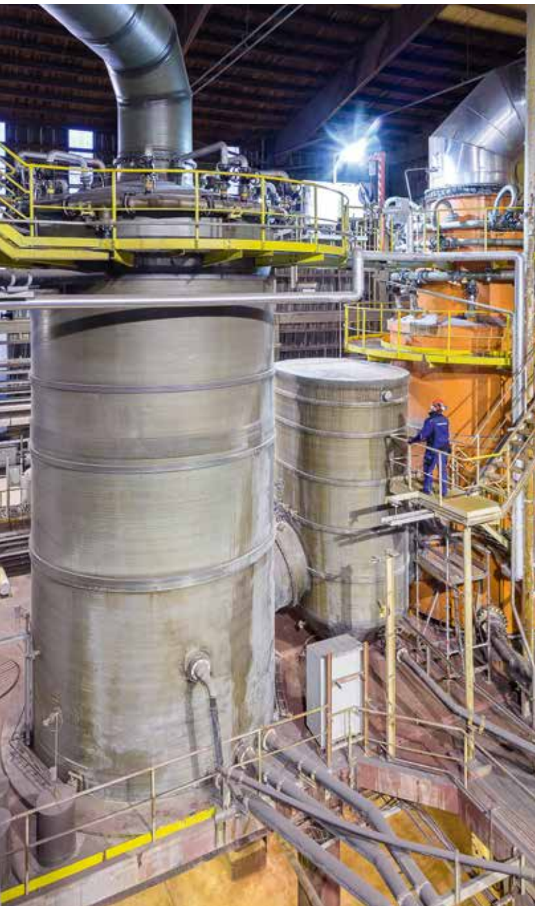
For the globally-active fertiliser manufacturer YARA, HUGO PETERSEN modernised the gas purification unit of the sulphuric acid plant at the site in Siilinjärvi, Finland.
