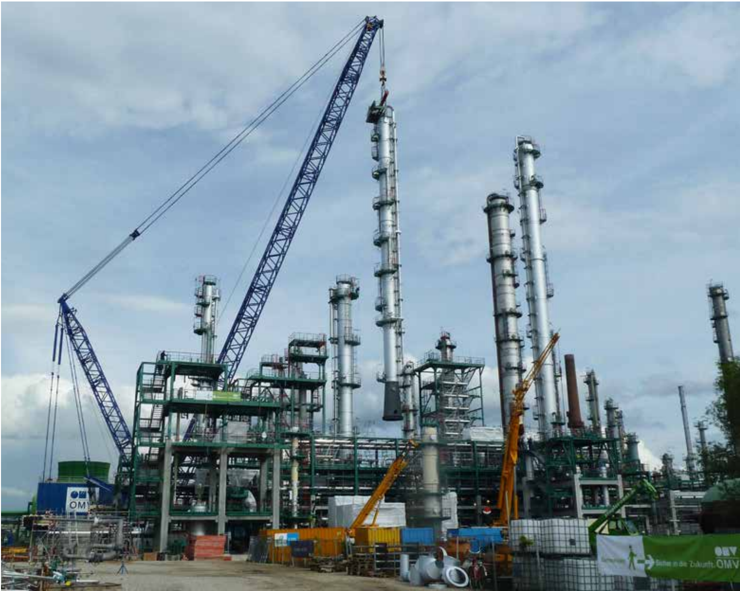
A crane with a load-bearing capacity of 1,250 tonnes lifts a column into place.
