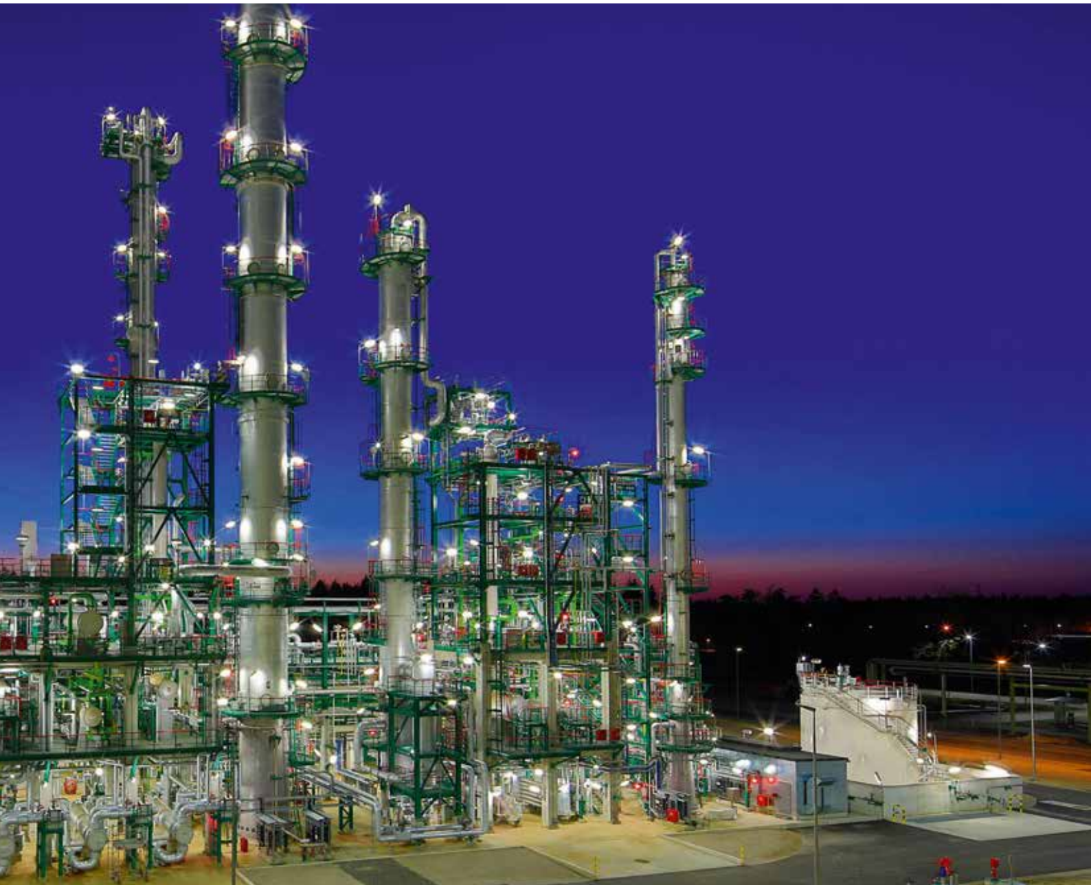
The butadiene plant at the Burghausen site has been producing consistently since spring 2015.
