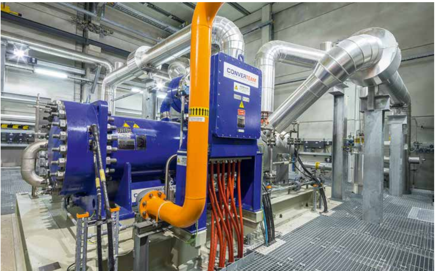
High-speed natural gas compressor with integrated electric motor and active magnetic bearings in a gas compression station.
