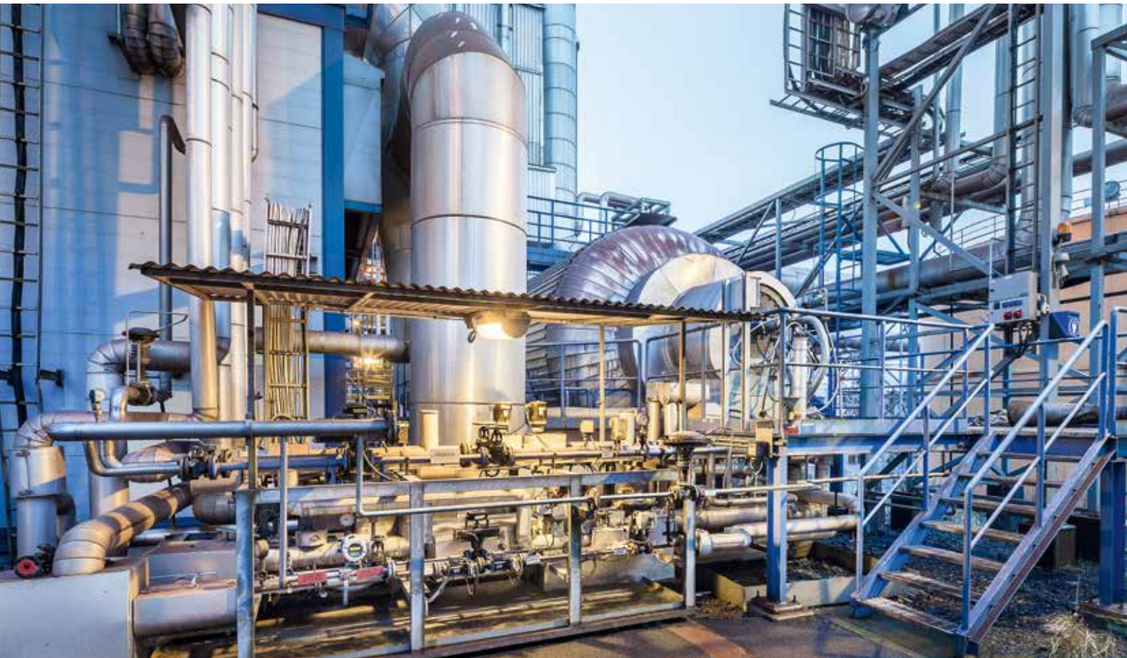
Also for YARA, at the Finnish production site in Siilinjärvi HUGO PETERSEN extended the existing sulphuric acid plant – for the purpose of increasing capacity – to include sulphur incineration.
