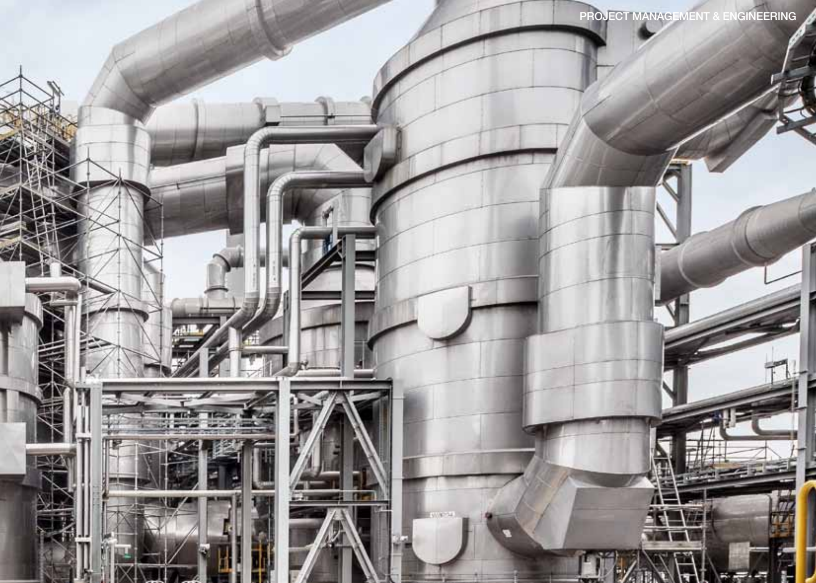
Partial view of a sulphuric acid plant
