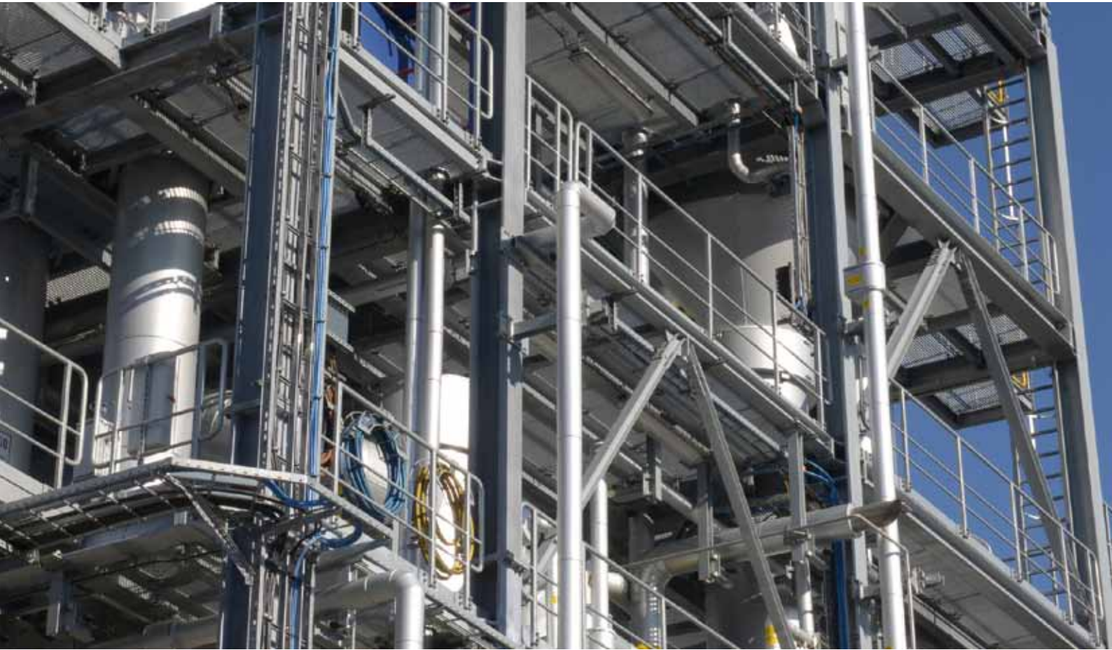
Evaporation plant EDA 2 in Schwarzheide
