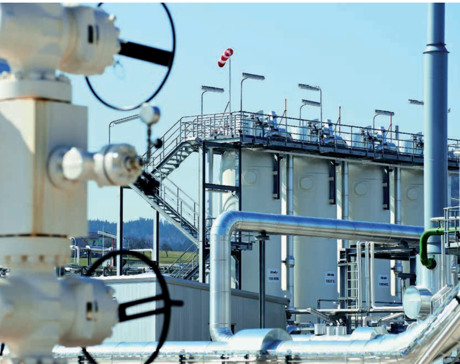
Natural gas storage facility Zagling
