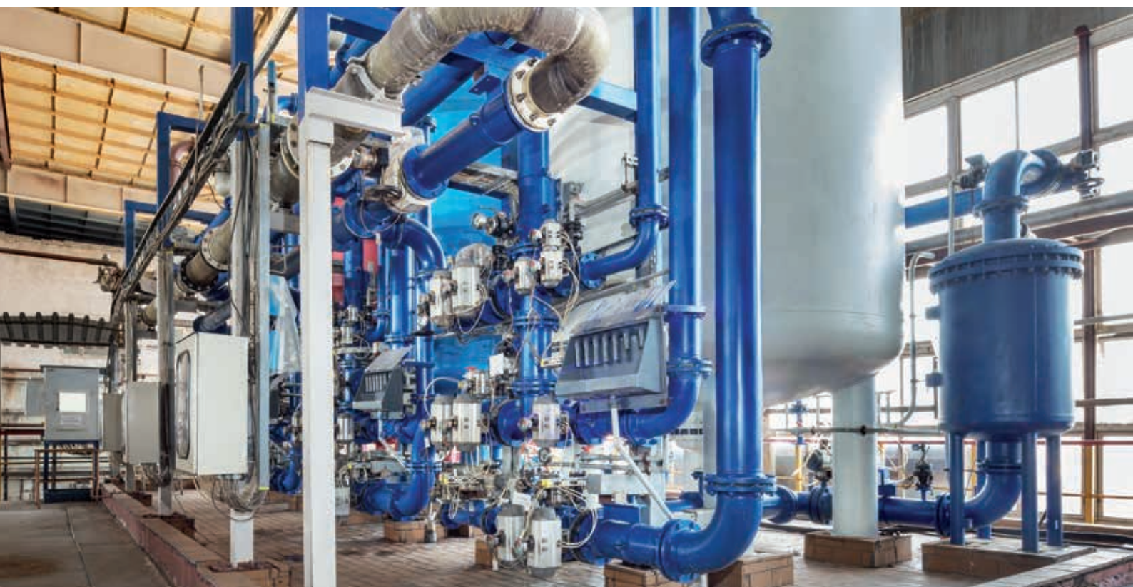
Part of an electrolysis plant
