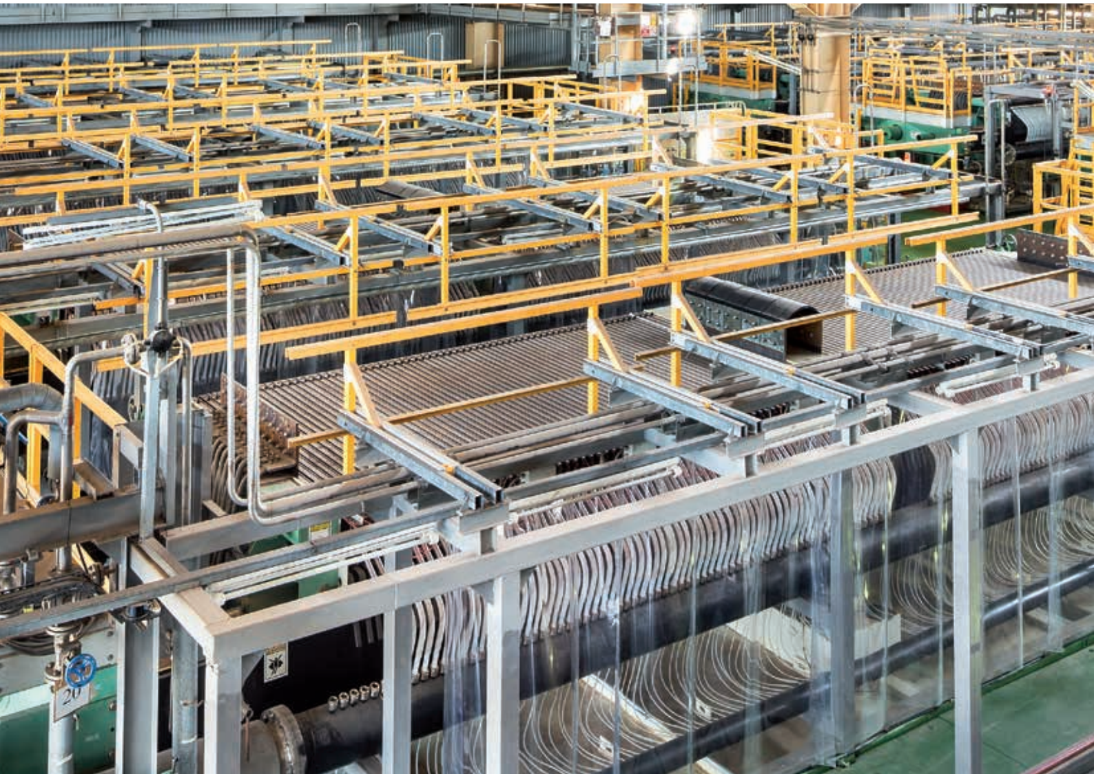
Cell room of a chlor-alkali electrolysis plant
